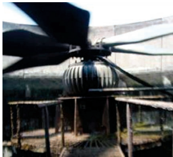
Cooling Tower Fan Gearbox
