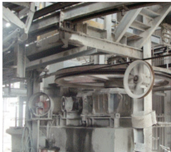
Conveyor Gear Box
