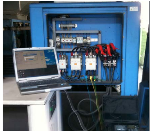
Checking electric consumption of air compressor.
